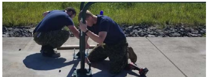
Capt Ovens, right, and Avr Hatch, left, fastening equipment to the apron.
