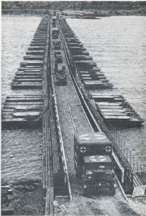
"MELVILLE" BRIDGE CARRIES TRAFFIC ACROSS THE RHINE This bridge across the Rhine at Emmerich, completed on 1 April 1945 by the 2nd Canadian Army Troops Engineers, is here seen from the right bank of the river.
