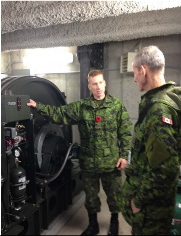
MCpl Larocque briefing BGen DesLauriers on the newly installed Airfield Arrestor System
