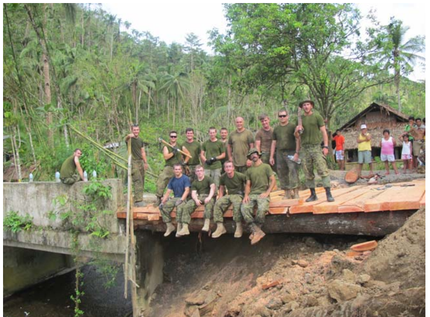
Members of the DART Engr Troop pose for a picture on the completed NSB in the municipality of Libacao.
