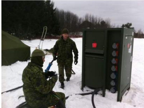
Cpl Kerr (electrical generating system tech) and Cpl Legendre (electrician), installing the power grid
