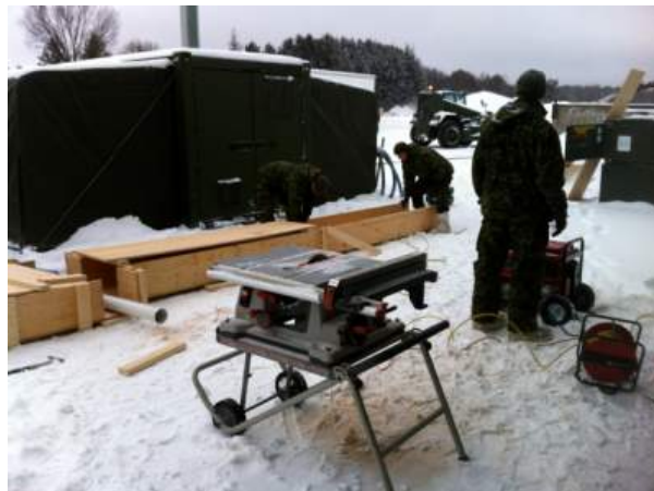
Carpenter at work, building a warm-air duct for pipes for MECCs used for ablutions
