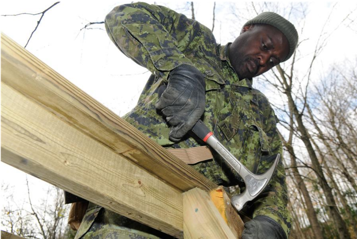
Cpl Hai Dai secures the bottom bracing during the refurbishment of the Mill Creek Bridge on the Trans Canada Trail near Ravenna, Ontario.
