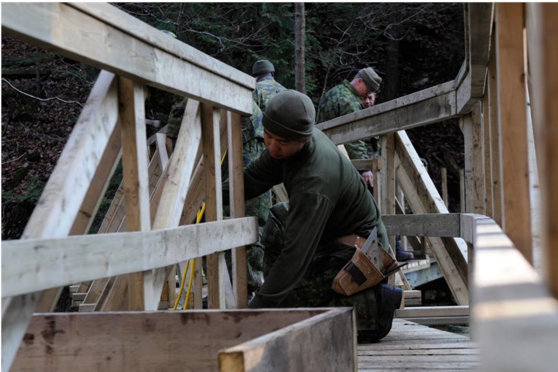
Sgt Andy Thomas puts the finishing touches on the handrail of the Mill Creek Bridge
